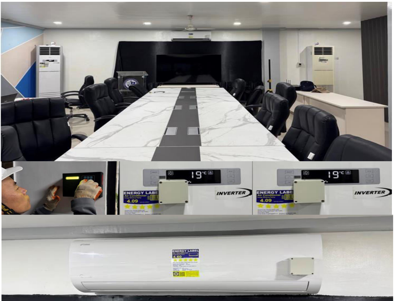
Fig 13. Finished SBMS Setup at NEMSU
